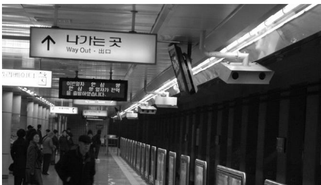
Fig. 4. Example of the installation of stereo cameras in the platform of some metro station
